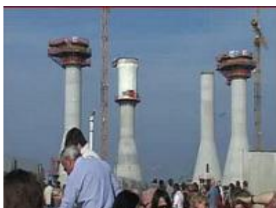
Fig. 3 5 MW offshore wind turbine (top), concrete foundations (bottom). Zeebrugge Belgium
